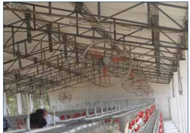
Figure 4. Stir fans and foggers increase air velocity within the house and create a cooling effect.
